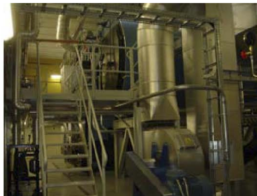
Part of the biofuel boiler in Arla-building.
