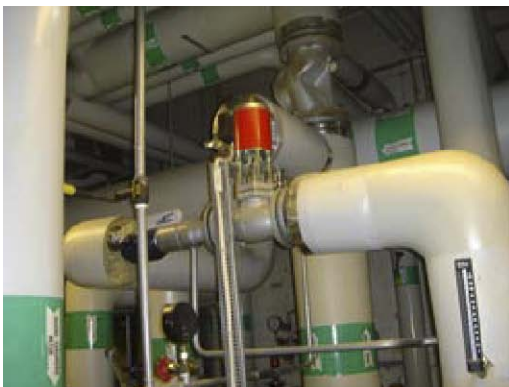
One of the efficient system valves.
