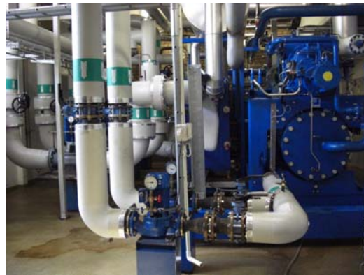
A forest of ducts and pipes carrying water of different temperatures in the cooling plant
