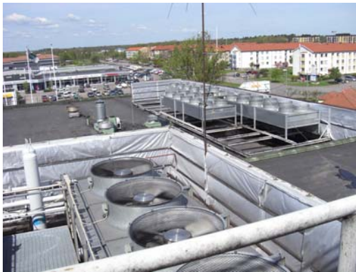
The outdoor coolers on the roof
